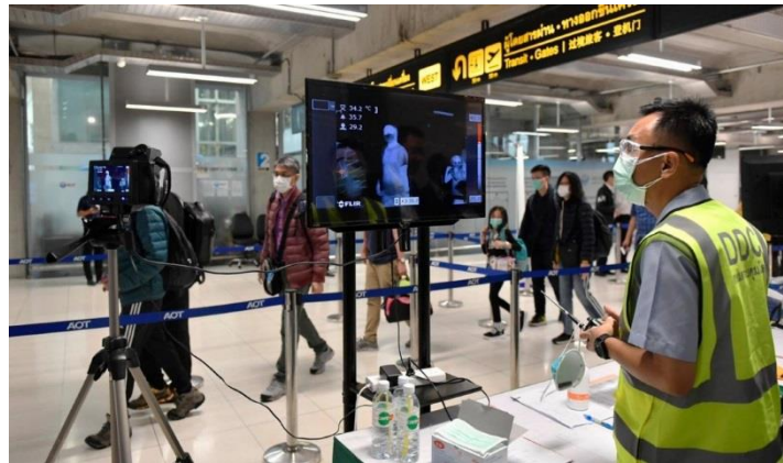
Figure 2. AI against Covid-19 Thermal camera installation at the airport
